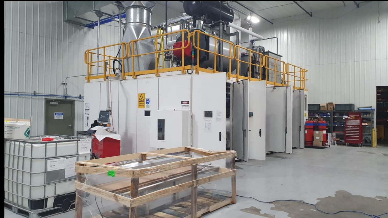
Picture of XTclave™ Recommissioning at US Facility
